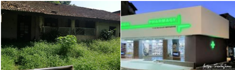
Figure 6. 25: Proposed development for the dilapidated building near Kahawatta Base Hospital and Education Resource Centre.
