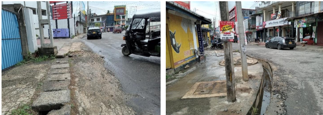
Figure No 3.1.1: Existence of improper drain network Source: Field Inspection , Urban Development Authority – District Office , Monaragala (2020)
