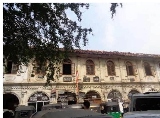
No Proper Maintenance
